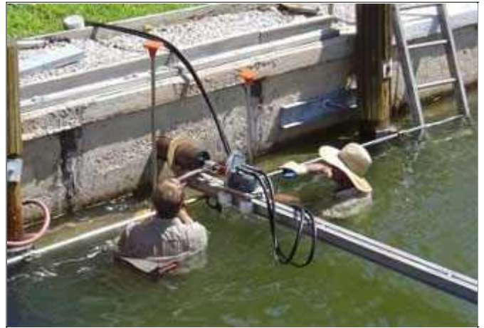
Submitted photo DSMS engineers start DSMS installation. Installations are performed from the water side of the seawall.
